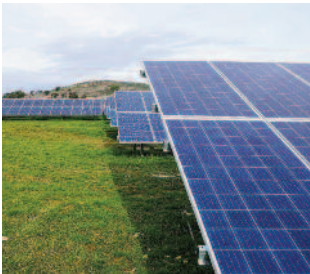
Indicative example of solar panels
